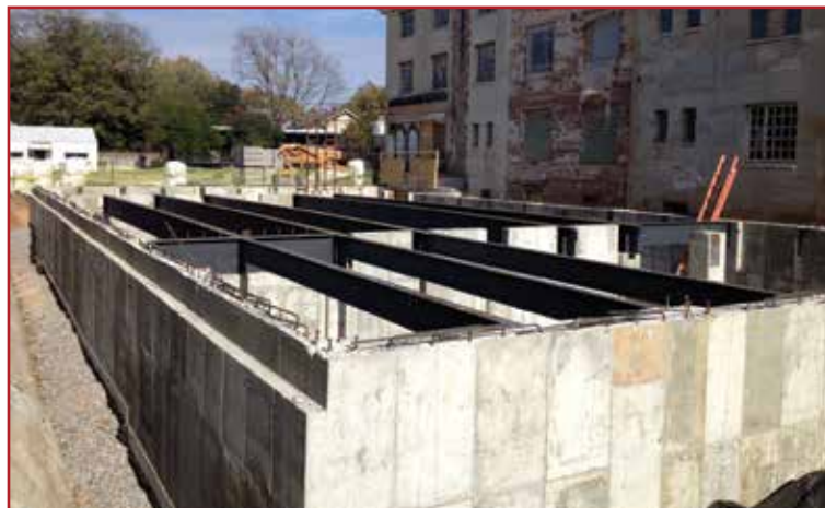
The basement foundation has been poured for the new addition that will house the study hall and new study rooms.
