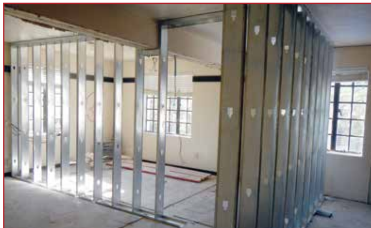
Stud framing is in progress on the second floor of the main house.
